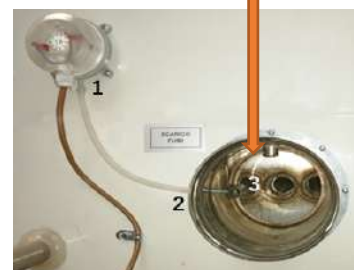
Fig. 7 pressure switch on flue
